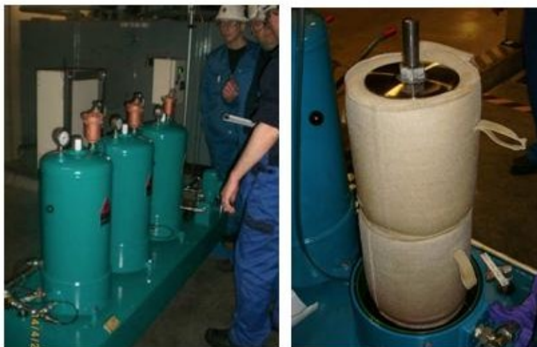
Illustration 12 – 13, shows the CJC PE conditioner unit, HDU 3*27/54 on a tank. Second photo is the used bags containing saturated ion exchange resins.
